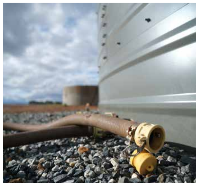
Image: Rainwater tank
