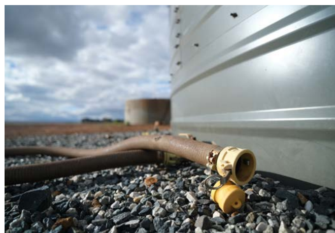
Image: Rainwater tank
